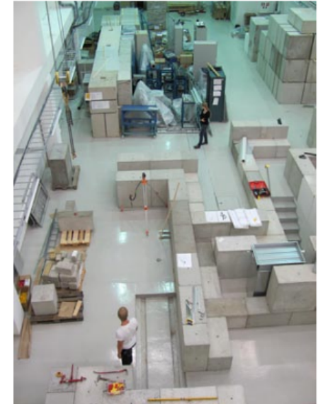
IGISOL components are waiting for the concrete walls to be built up in the new experimental hall.
